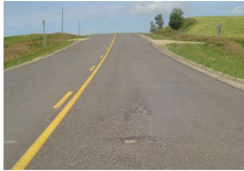
"Aging Asphalt Highway" A road that needs accelerated maintenance before it begins to fail – a common need in SD.
